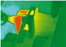
Motor: Bearing Problem
