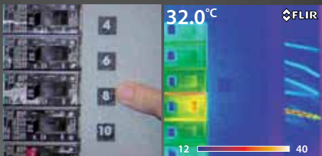
Bad connections are invisible to the naked eye but are clearly seen on the thermal image.
